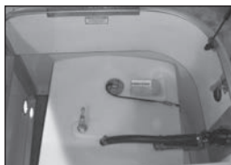
Frequently Inspect Hoses & Clamps for Fuel Leaks.
